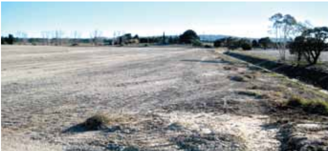
Dux Moss Vale containment cell being constructed (above picture) and the finished remediated area (below picture)
