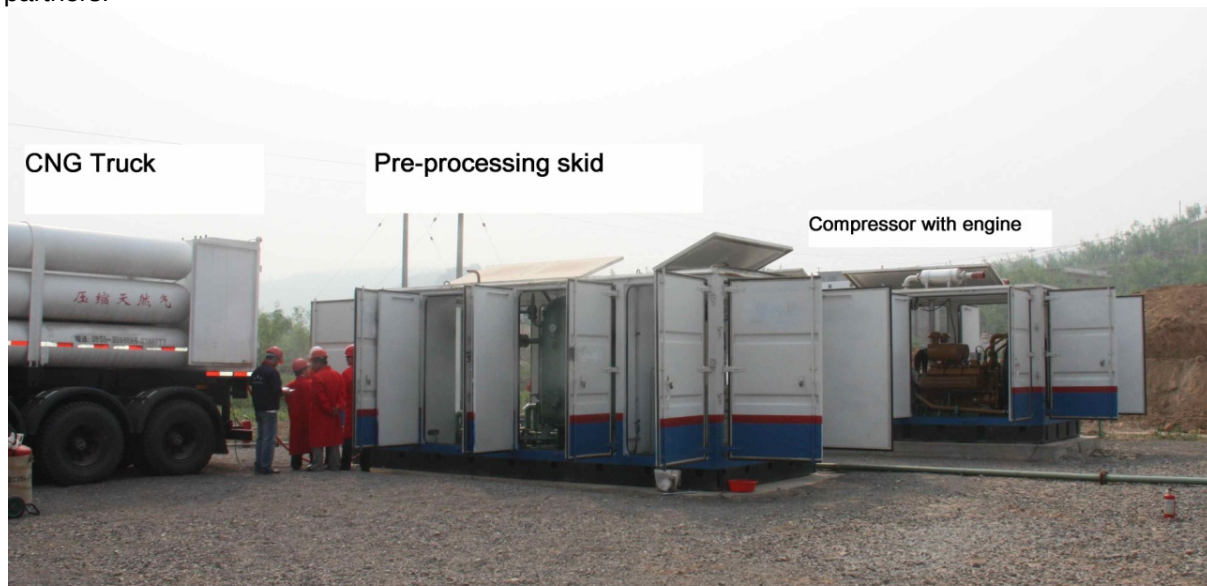
Compressed Natural Gas (CNG) facilities - Shanxi Province, China. Sino Gas anticipates using facilities similar to these for its Pilot.
