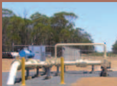
Berwyndale Wallumbilla Pipeline
