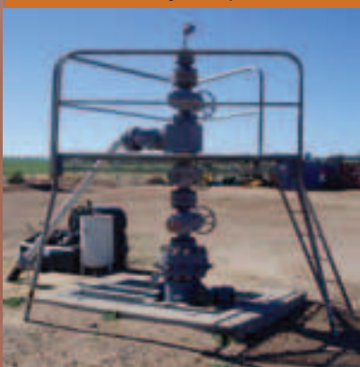
Mondarra Gas Storage facility
