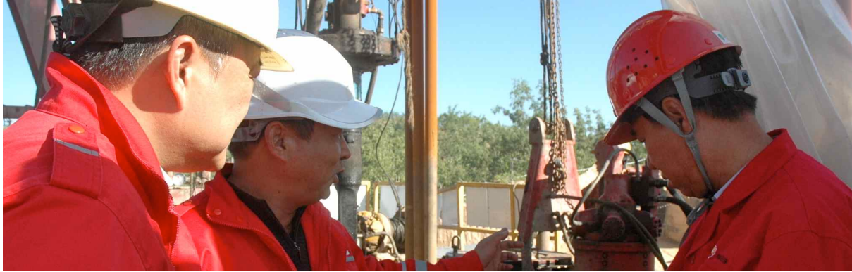
Sino Gas's Scott Li and Larry Yuan (left) supervise operations on the TB08 well
