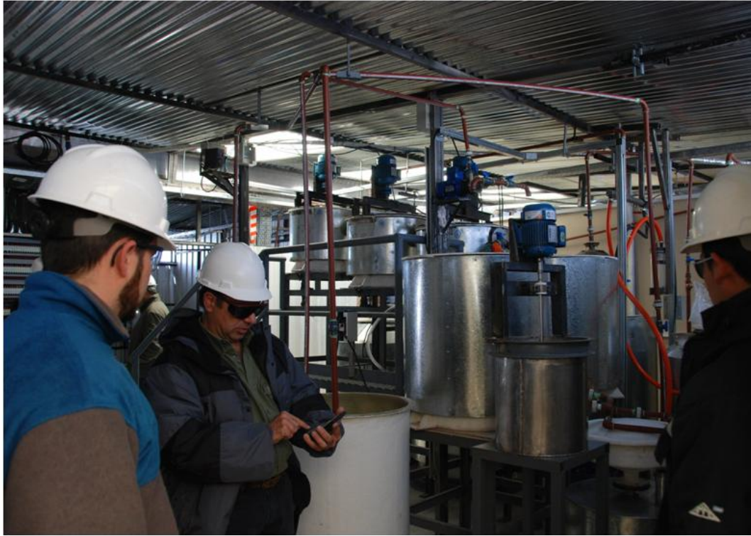
Pilot Plant Facilities at Salar de Olaroz
