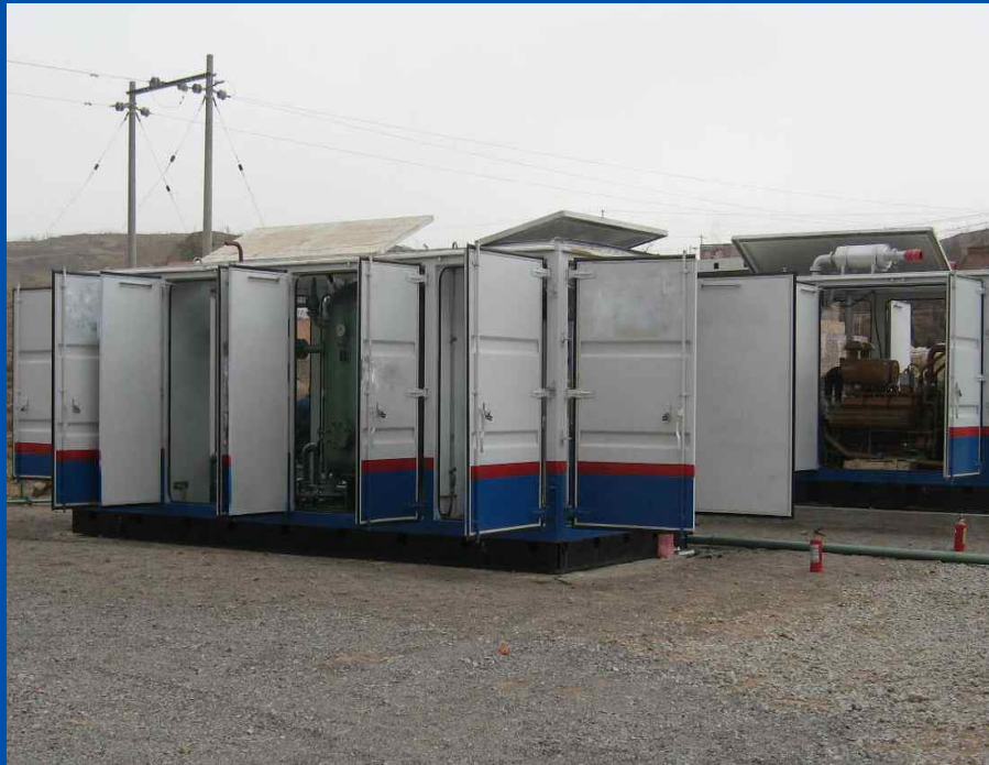
Pilot Station – Example of Modular Equipment
