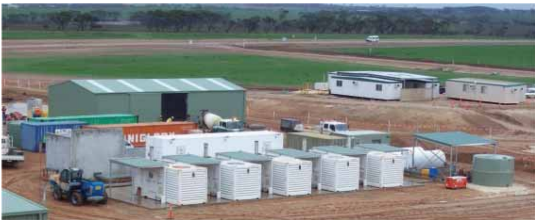
Figure 8.10 View of Power Station Generators, with ferro-silicon storage shed behind.
