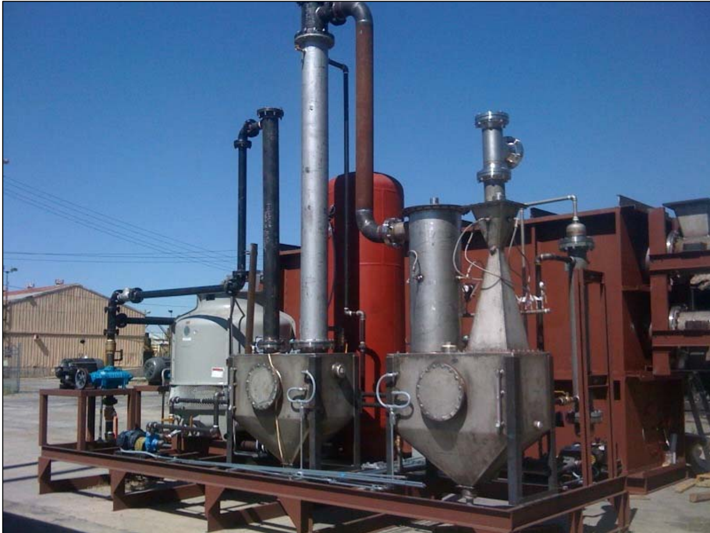
0.5 TPH Prototype Gasification Unit with First Stage Gas Clean Up
