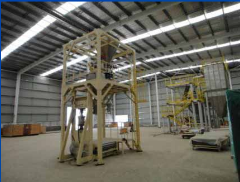
Installed bulk bagging machine
