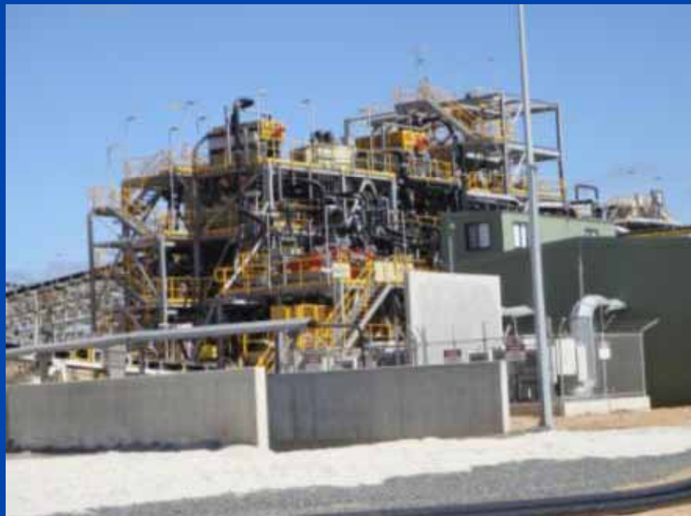
Heavy media plant and spodumene stockpile area
