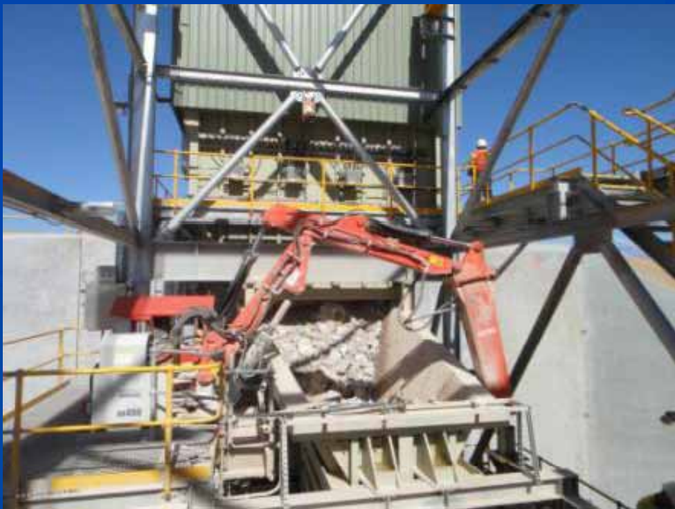
Feeder to primary crusher
