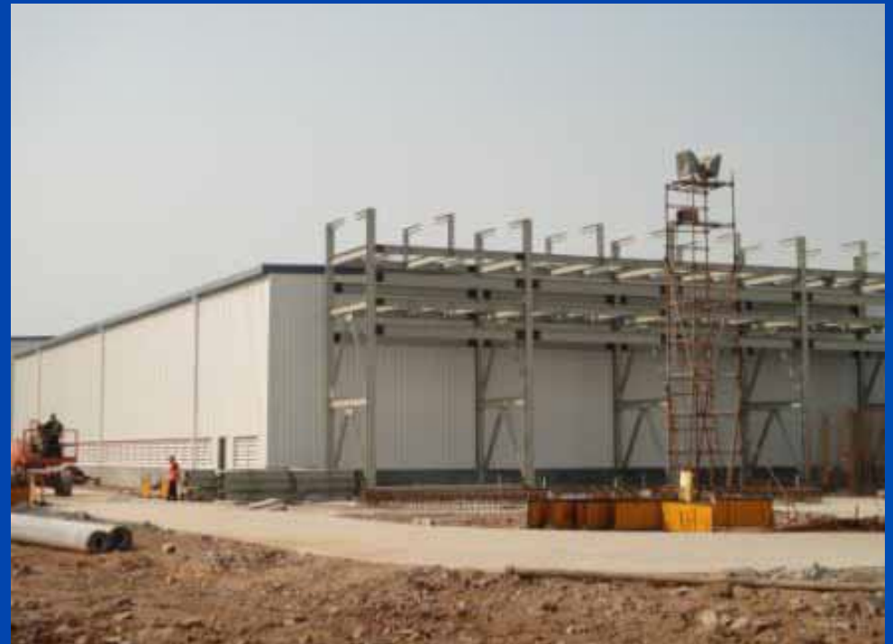
Warehouse and pipe rack
