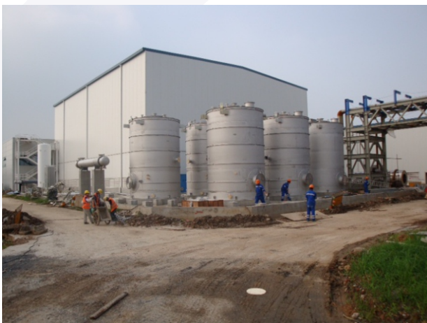
Purification Area - Jiangsu, China
