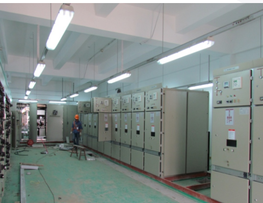
High Voltage Room - Jiangsu, China
