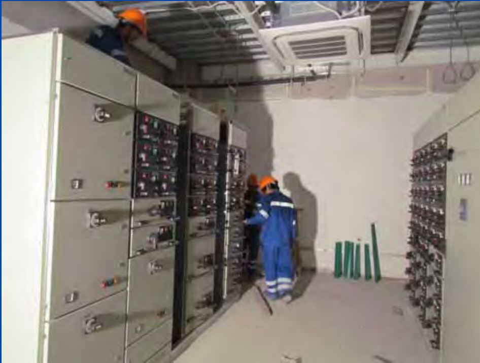
High Voltage Room
