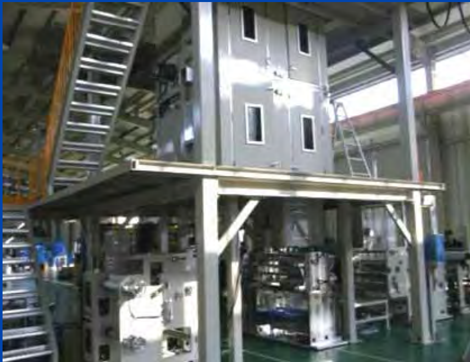
KUBT separator formation machinery
