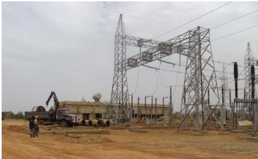
Sikasso Substation Feb 2011
