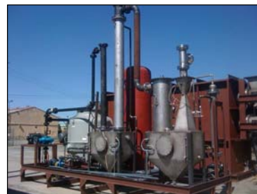
0.5 TPH Prototype Gasification Unit with First Stage Gas Clean Up (ARE)
