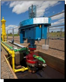
Recent Gas Production Well Head
