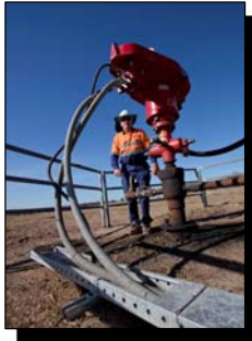
Renovated Meridian Seam Gas production well
