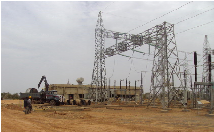
Sikasso Substation Feb 2011
