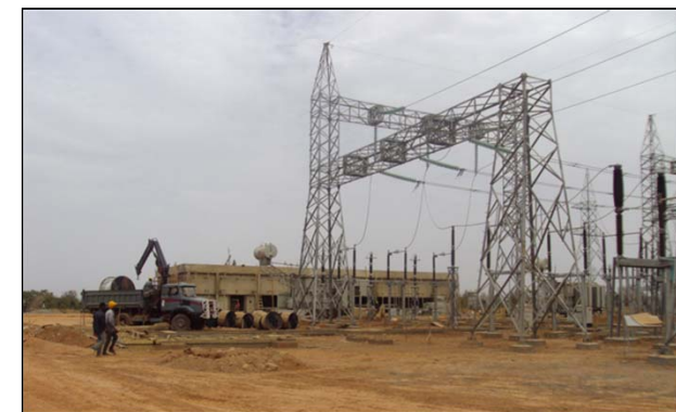
Sikasso Substation Feb 2011
