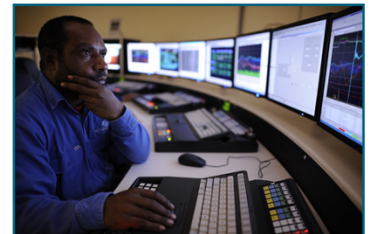
New Control Room at CPF began operating in January 2012
