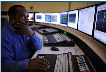
New Control Room at CPF - commenced operations in January 2012
