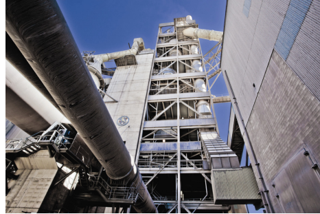
Birkenhead plant, South Australia
