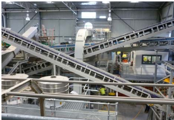
3. Interior of Materials Recovery Facility (MRF) building, with control room on the right
