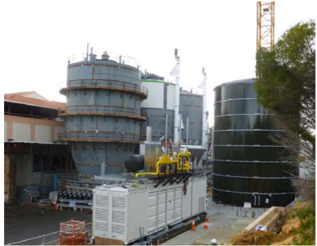
2. DiCOM bioconversion vessels with anaerobic liquor tank and power generation unit in foreground
