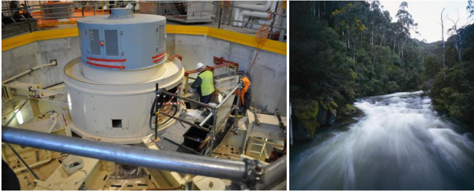
Hydro power station
