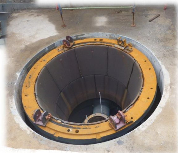
Gyratory crusher unit base Source: BBY 22/06/2012
