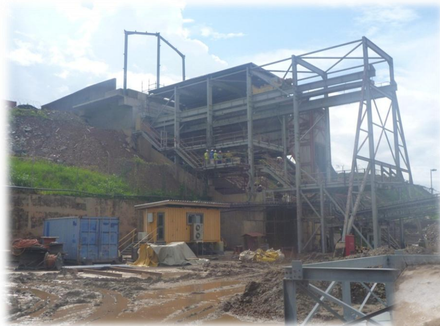
Crusher infrastructure Source: BBY 22/06/2012
