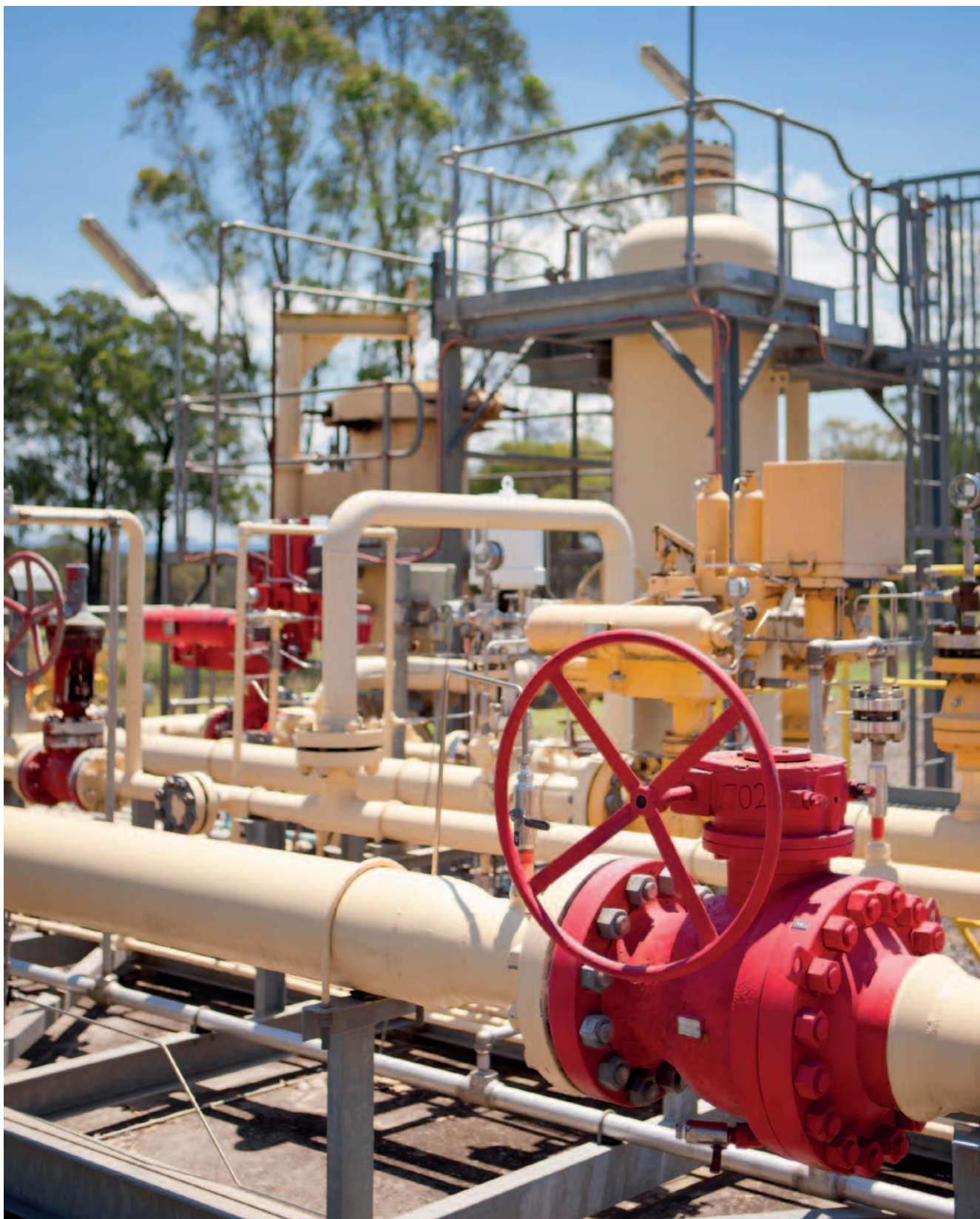
Wilton Meter Station, New South Wales
