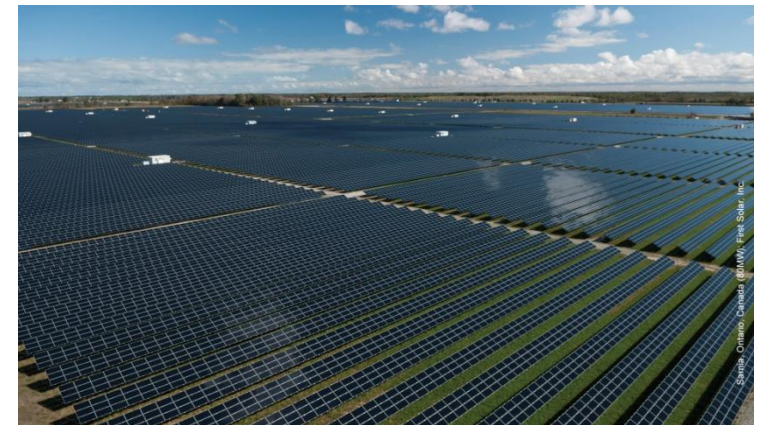
Sarnia Solar Farm, Canada, 80 MW
