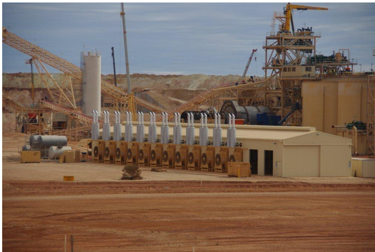
Power plant at Garden Well
