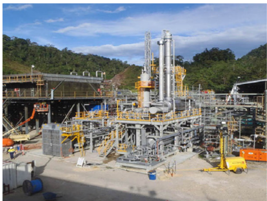
TEG Dehydration Unit - operational
