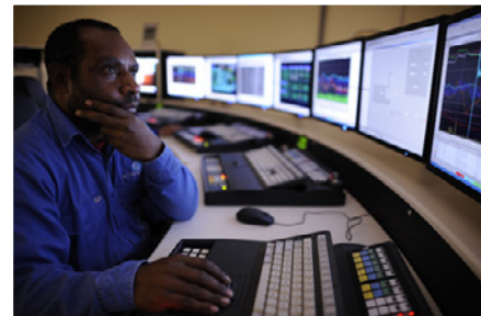
New CPF Control Room - operational
