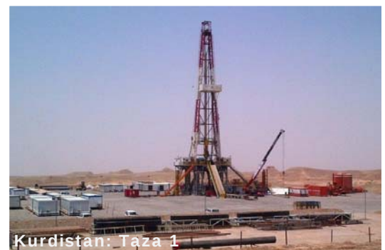
Central Processing Facility
