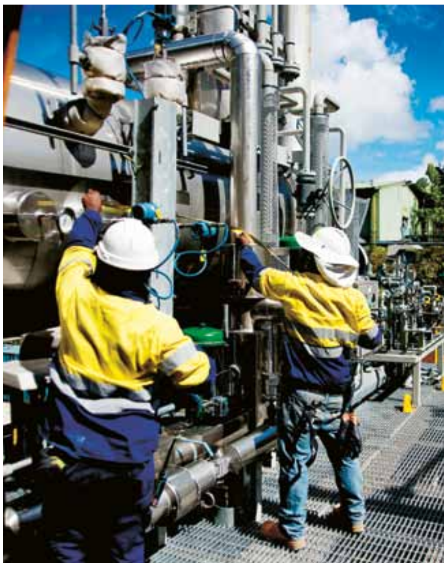
New Tri Ethylene Glycol unit at the Central Processing Facility, PNG Highlands
