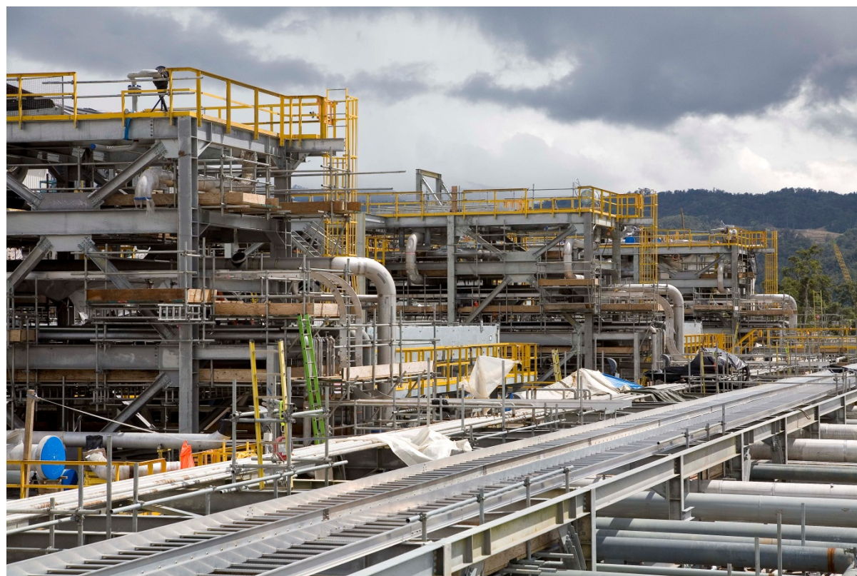
Hides Gas Conditioning Plant, June 2013.
