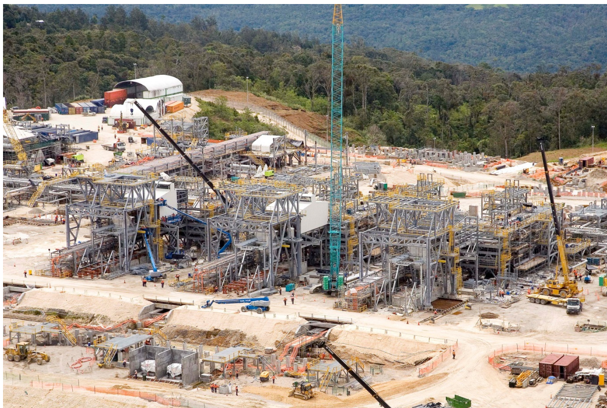
Hides Gas Conditioning Plant, May 2013.
