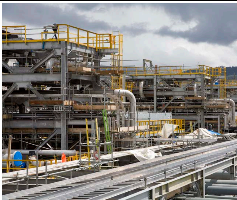
Hides Gas Conditioning Plant, June 2013
