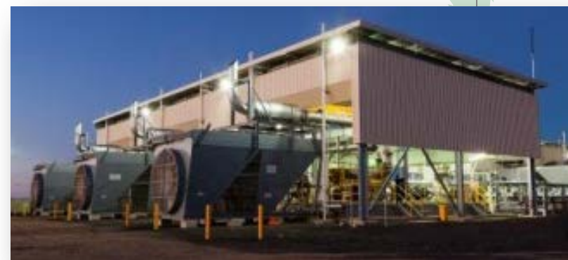
Wallumbilla compressor station on the SWQP
