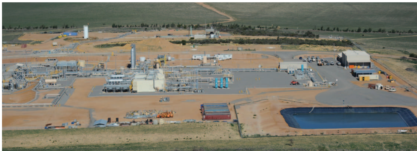
Capital expansion works recently completed at the Mondarra Gas Storage Facility have increased the storage capacity fivefold to 15PJ.
