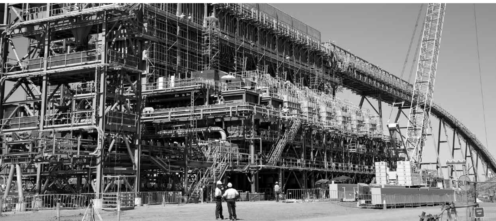
Monadelphous at a screenhouse facility at an iron ore operation, Cape Lambert, Western Australia.
