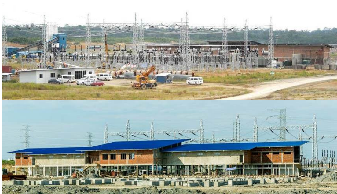
275kV Main Substation
