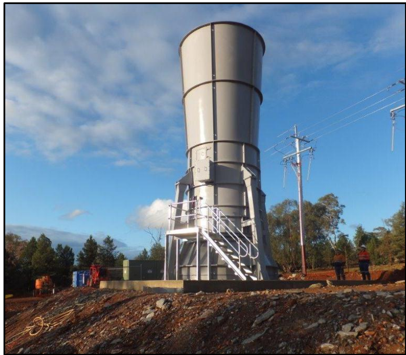
Primary Vent Fan commissioned Oct 2013
