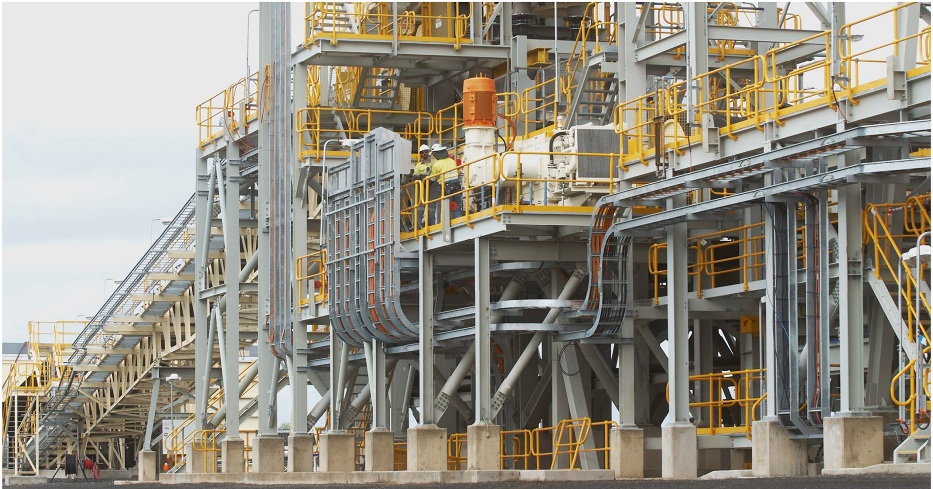
The drift conveyor drive station, Rio Tinto Kestrel Mine Extension, Queensland.
