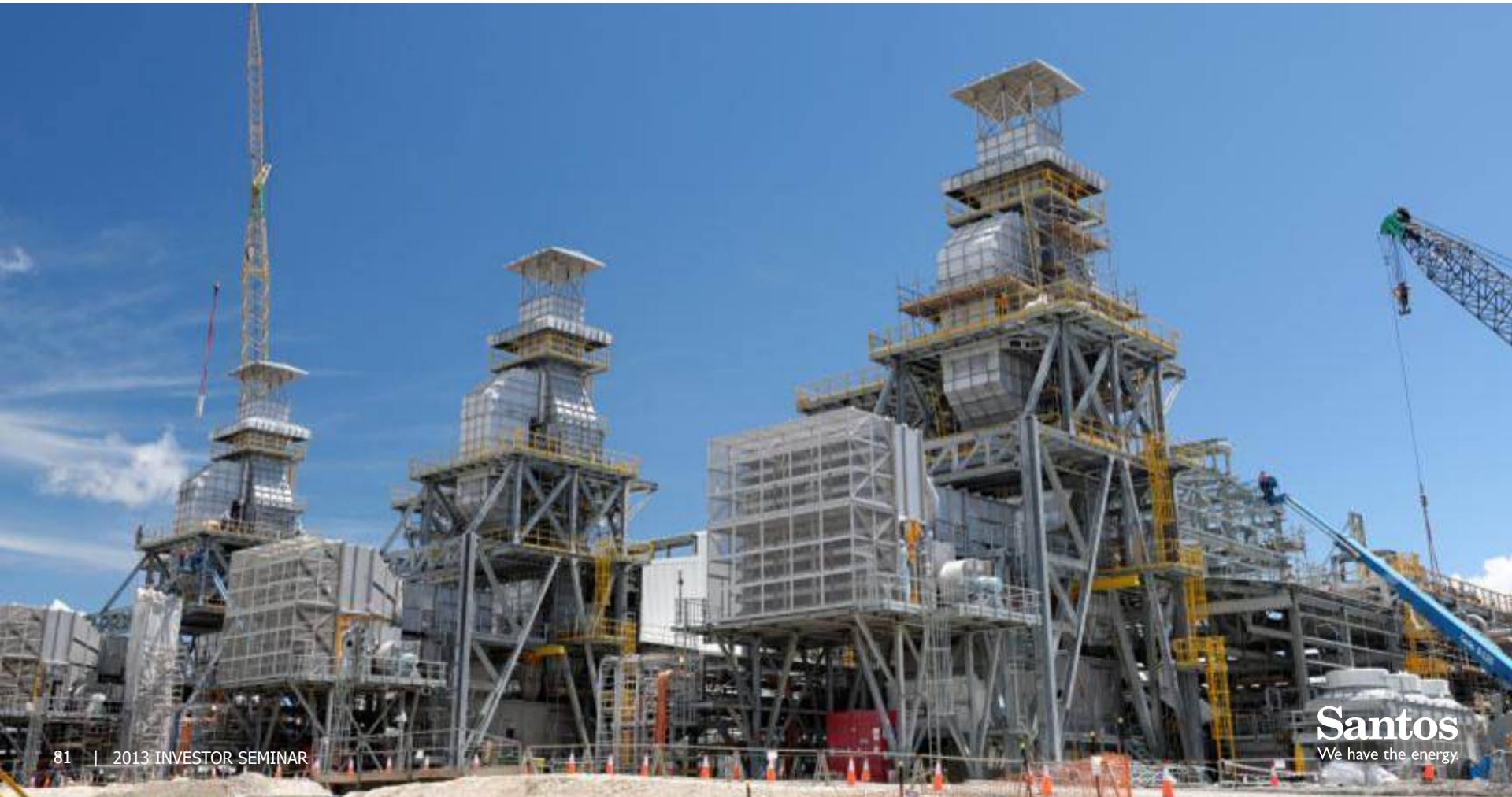
Hides Gas Conditioning Plant
