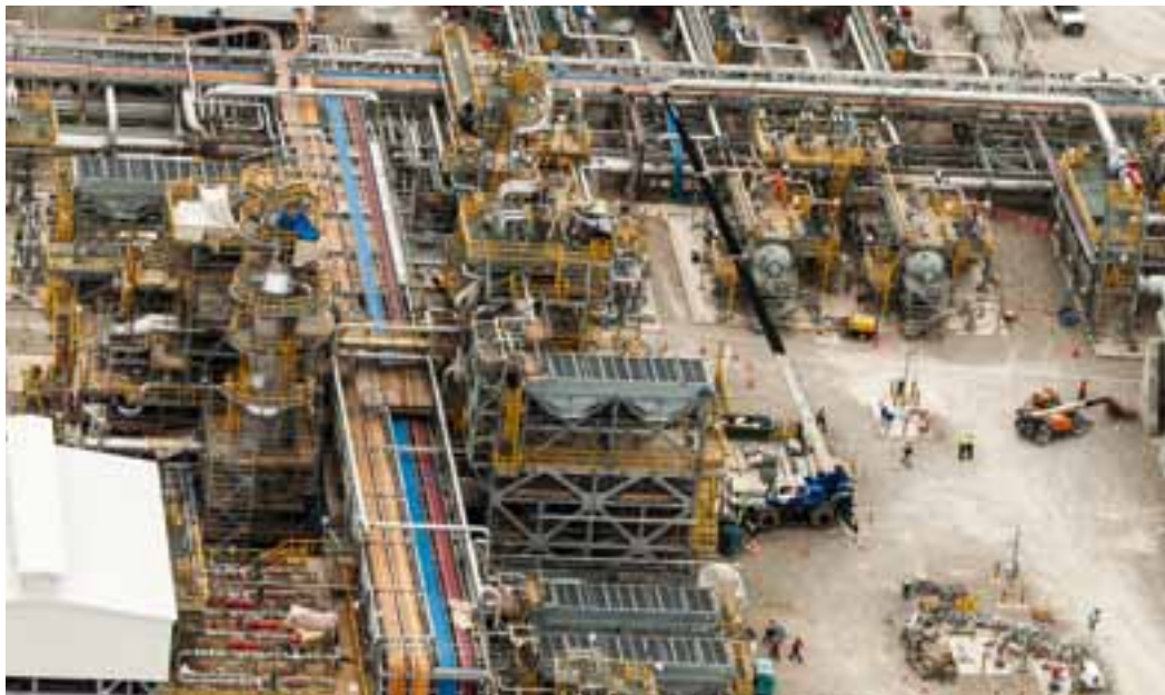
HIDES GAS CONDITIONING PLANT. PNG Highlands.
