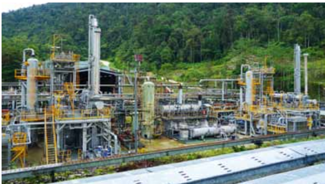
TRI ETHYLENE GLYCOL (TEG) DEHYDRATION UNIT. Central Processing Facility, PNG Highlands.
