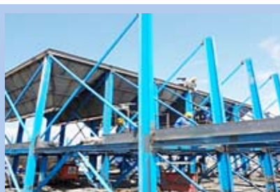
Furnace dedusting installation
