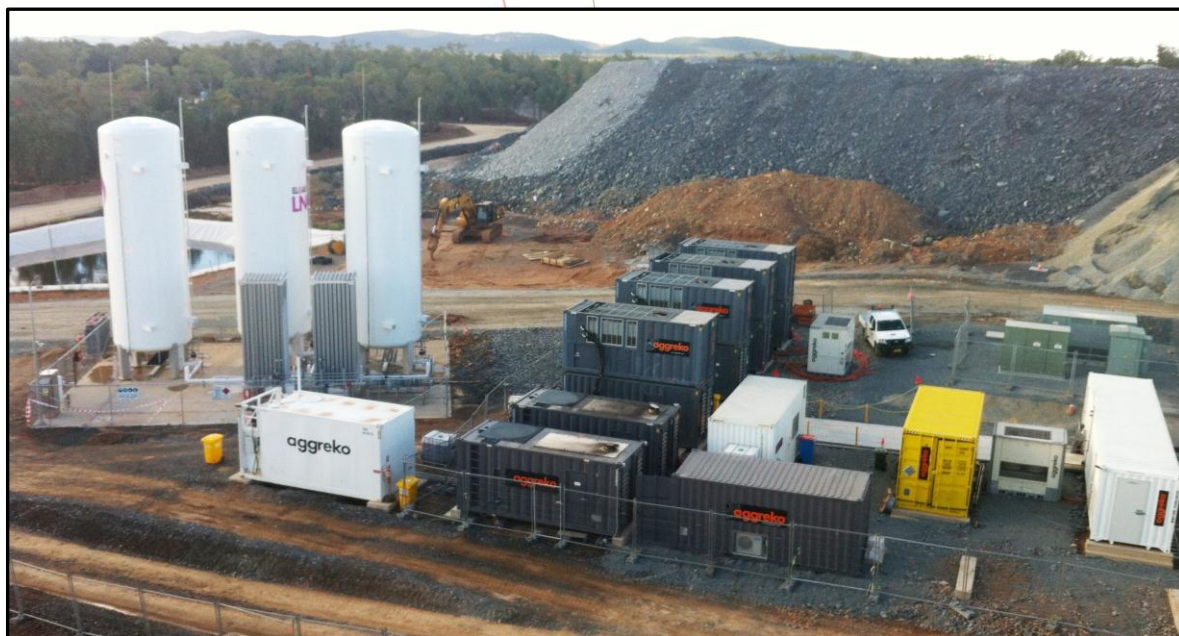
Completed LNG fired power station
