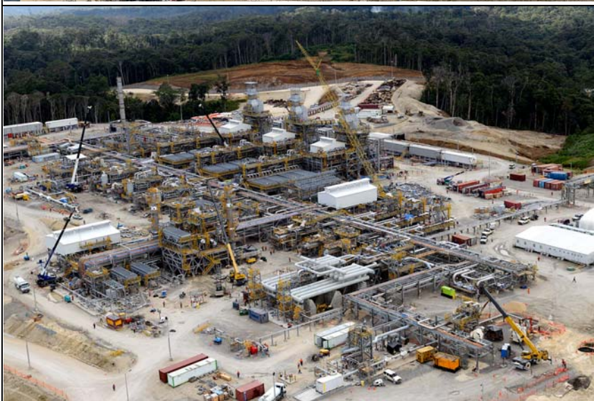
Hides Gas Conditioning Plant November 2013
