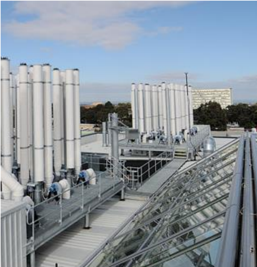
150 exhaust fume stacks were installed on the Monash University, New Horizons Building.
