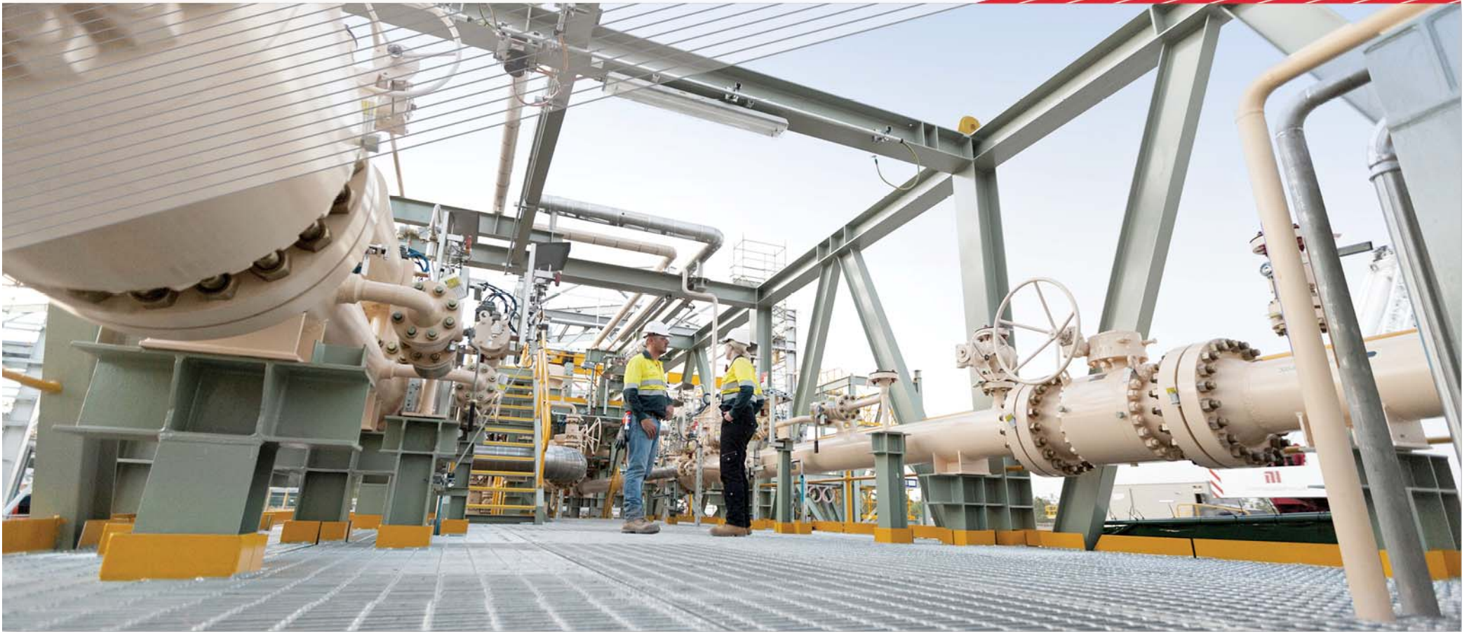
Origin Energy, Talinga Pipeline Compression Facility Project, Condamine, Queensland
