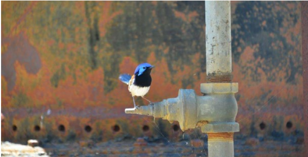
Image: Part of the original Tocabil pump station
