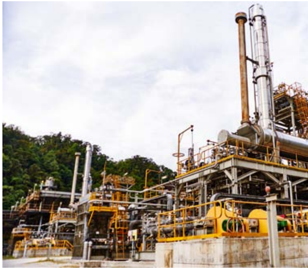
ABOVE: Tri Ethylene Glycol (TEG) Dehydration Unit, Central Processing Facility, PNG Highlands.
