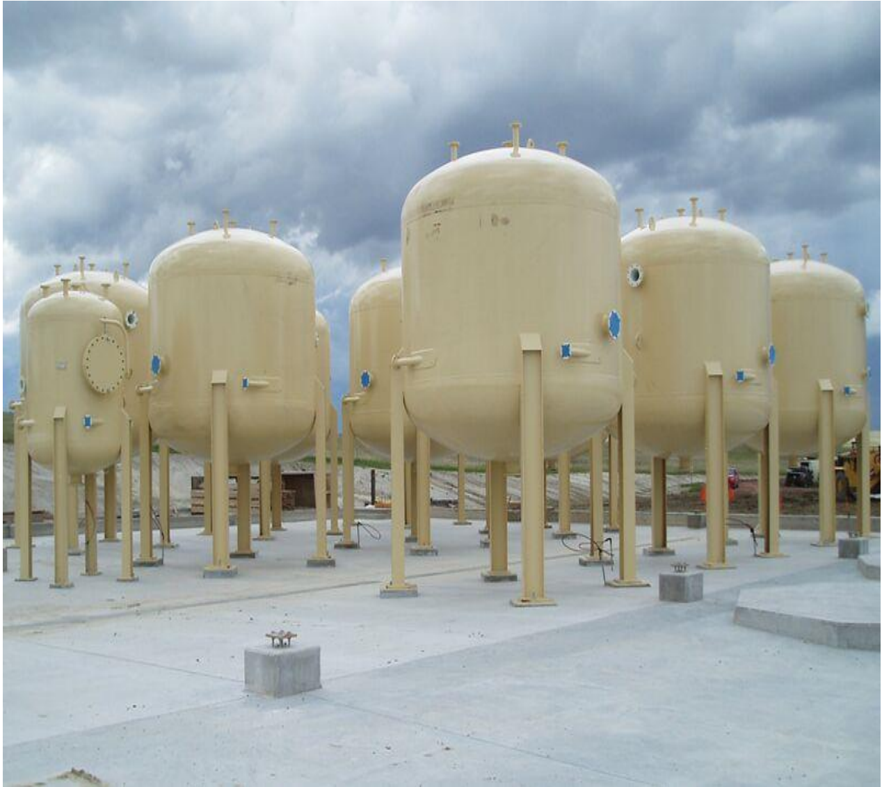
Figure 3: Ion exchange columns and pressure vessel tanks installed in CPP
