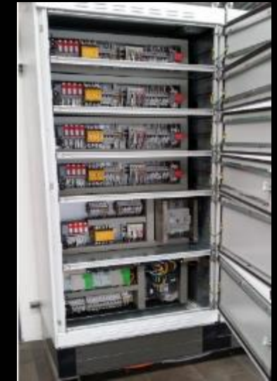
Failsafe Instrument Cubicle (FIC)
