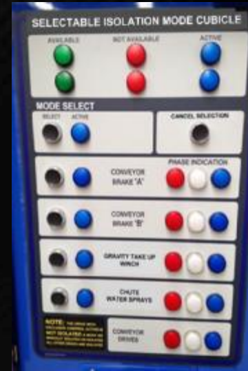
Selectable Isolation Mode Cubicle (SIMC)
