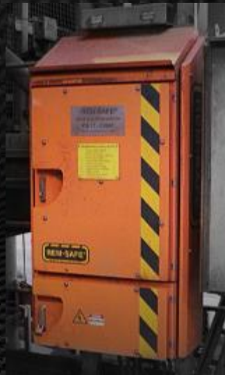
Field Isolation Station (FIS)
