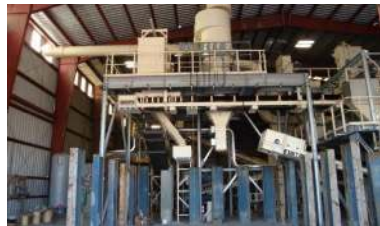
Optical Sorting, Screens, Magnets, Eddy Current, Crushers
