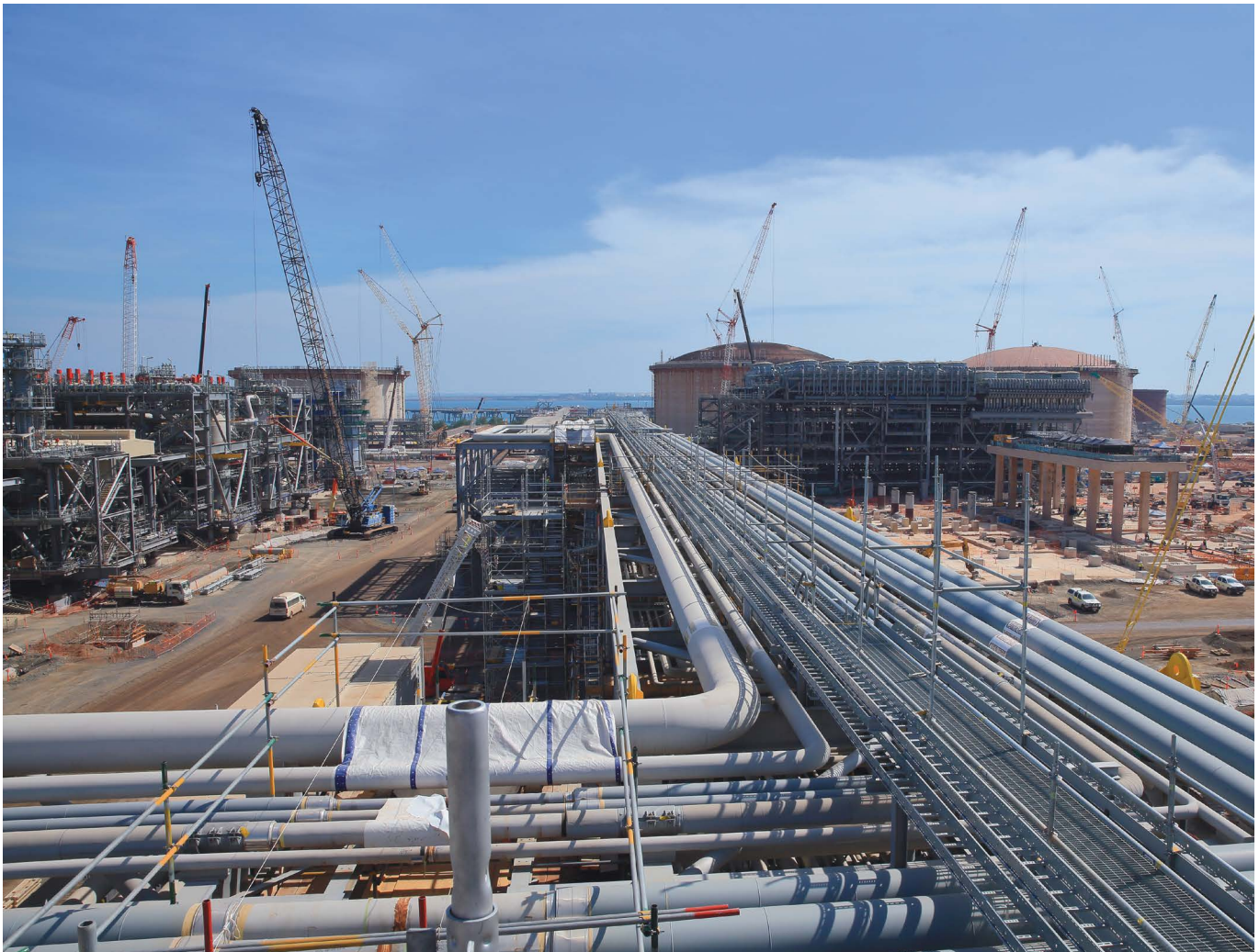
Top Overlooking by-pass module and slug catcher vessel at Spring Gully Pipeline Compression Facility, Roma, Queensland (photo courtesy of Australia Pacific LNG)
