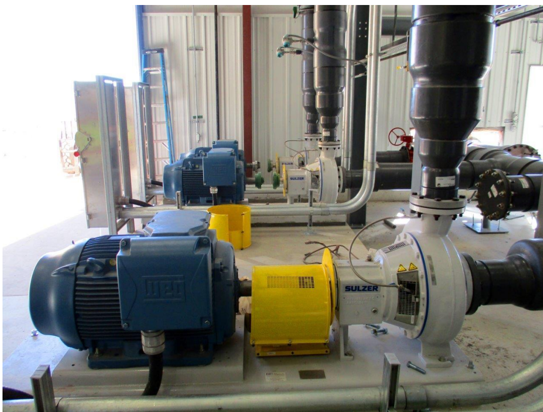
Figure 4 : Installed Pumps in the CPP, Lance Projects – 13 October 2015
