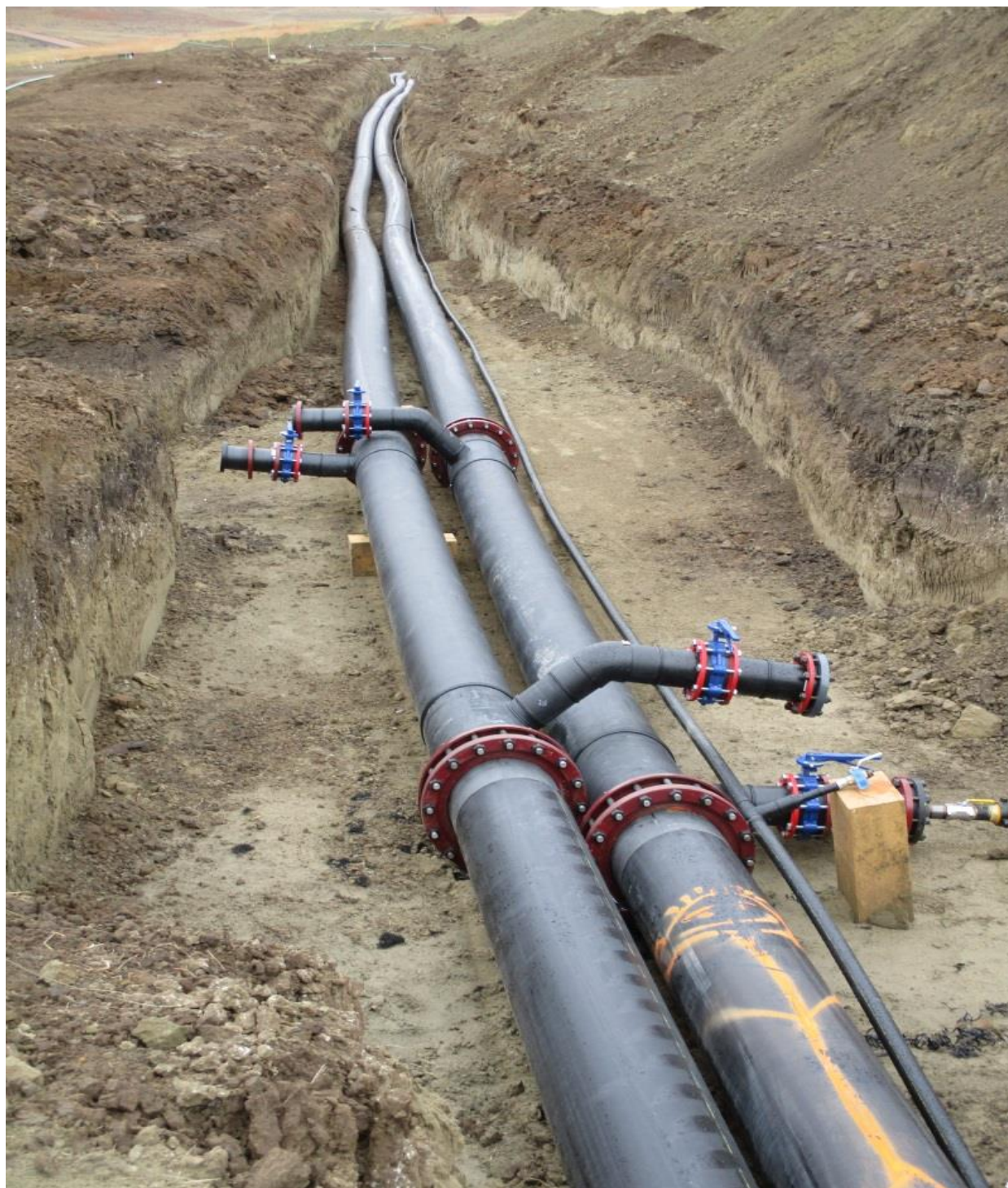
Figure 5: High Density Large Diameter Polyethylene Trunklines from CPP to Well Fields, Lance Projects – 28 September 2015
