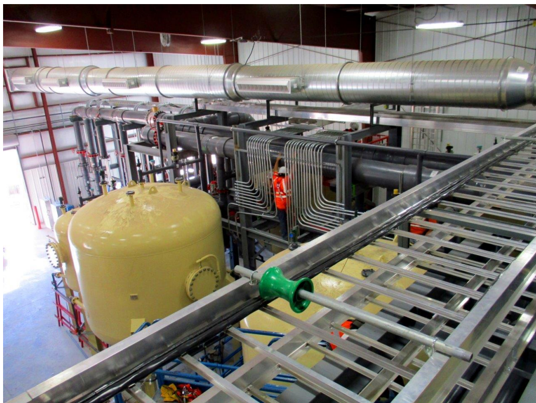
Figure 3 : Installed Ion-Exchange Vessels in the CPP, Lance Projects – 13 October 2015
