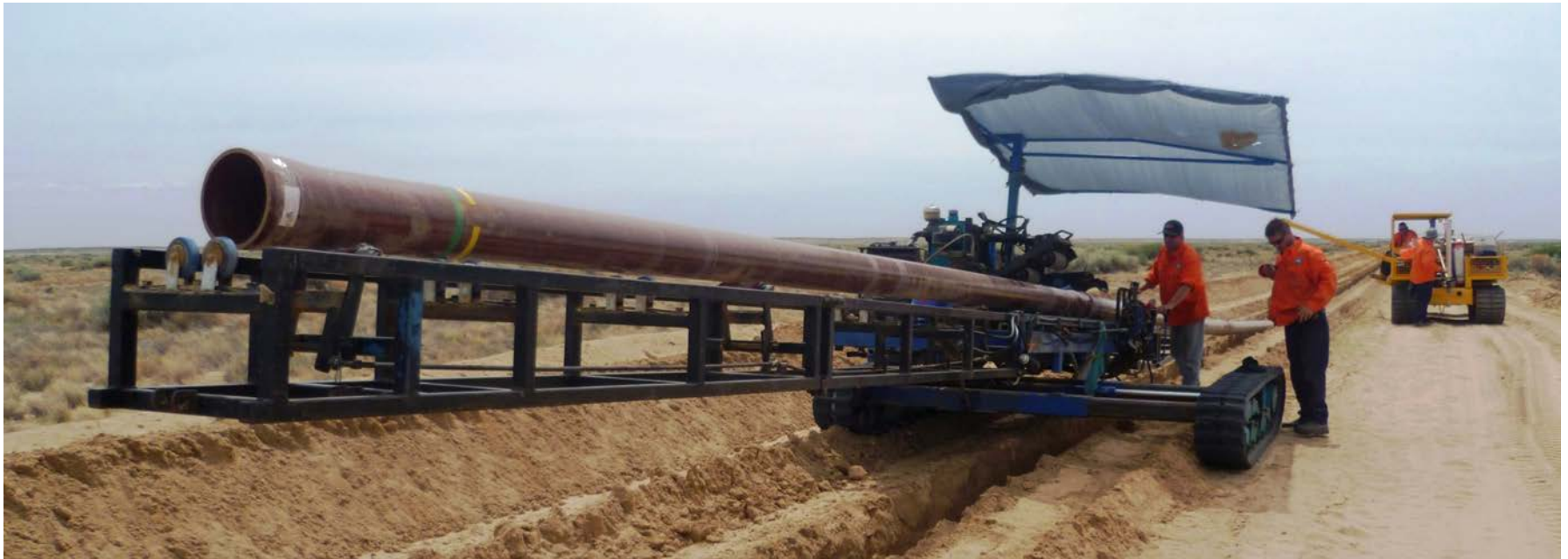
Pipe assembly of 200 nominal bore Lycium to Moomba pipeline with hydraulic spinner
